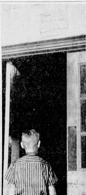
This door at Midwood School was propped open by the Bureau of Fire Prevention. The sign over the door reads, "Please! Keep Doors Closed" and is signed by the Bureau of Fire Prevention.
