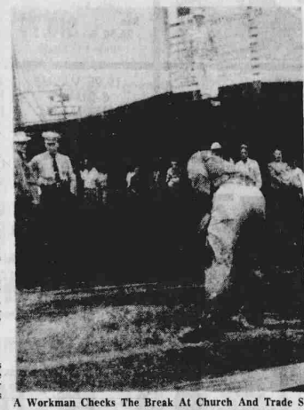
A Workman Checks The Break At Church And Trade Sts.
